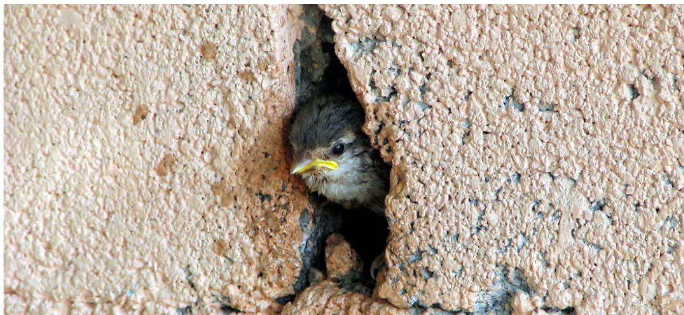
Figure 1: Bird peering through the crack of a building. Image cropped from original by Eperales, licensed under CC by 2.0
